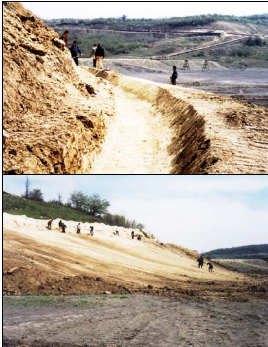
Photos 3 and 4 Preparation of the subsoil prior to the installation of the GCL
