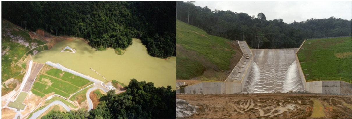
Photo 4: Santong #3 sediment control structure.
