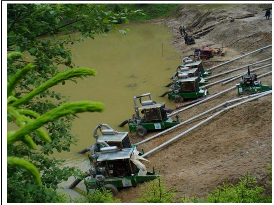
Figure 6. Mitigation measures in order to evacuate the excess water from the top of the Tarnicioara tailing dam
