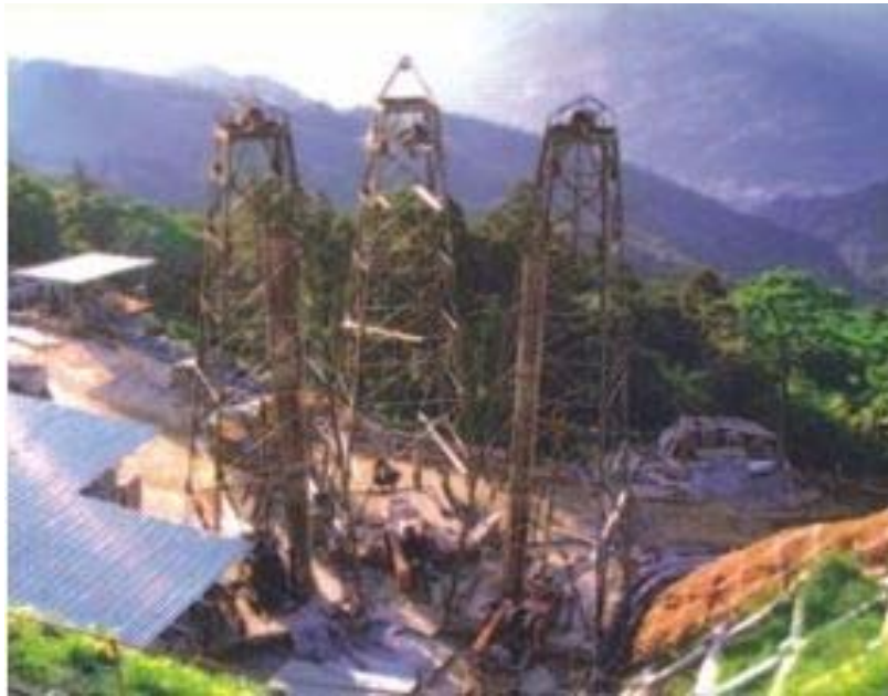
Fig. 4. Arrangement of drill rigs on the ground surface for drilling vertical grouting holes around Exhaust Shaft №1 of Pin Lin Tunnel
