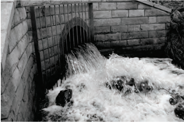
Figure 4 Engineered gravity discharge pipe at Page Bank
