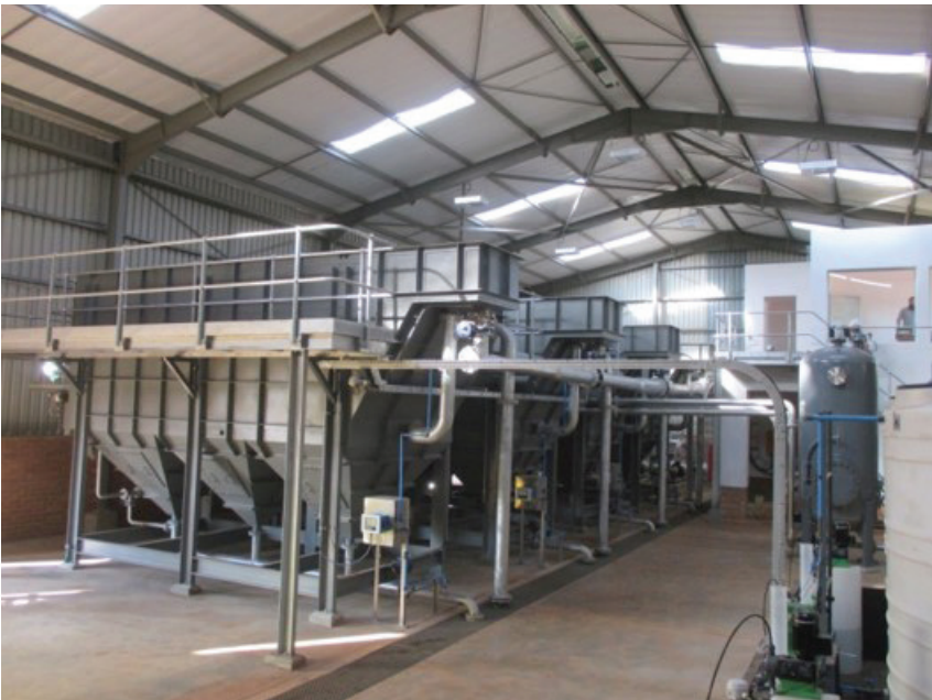
Figure 1 – Dissolved air flotation units inside the WRP
