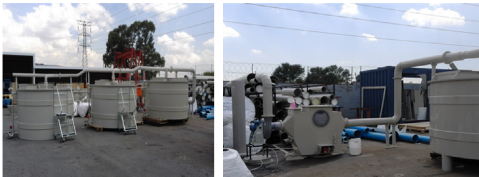
Figure 4 Biological sulphate reduction pilot plant, showing the reactors (left) and the gas scrubber (right)
