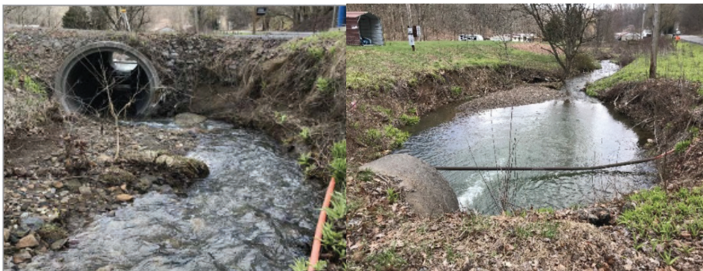
Figure 3 Obstructed Conditions at an Undersized Culvert Inlet (Left) and Outlet (Right)
