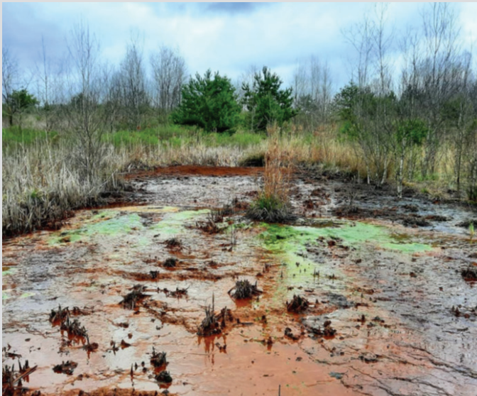
Figure 3 The "Volcano Seep" discharges from the toe of a previously reclaimed area that now shows clear evidence of infiltration and erosion. This is a planned site for future reclamation
